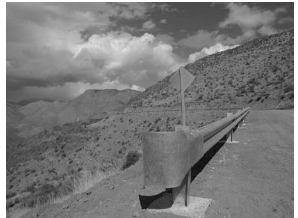
Figure 5: Part of several kilometers of the new (and much appreciated) guardrail installed on the road to Cerro Pachón.
