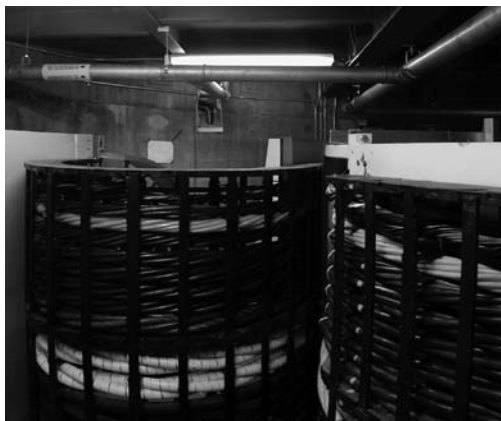
Figure 3: Azimuth cable wrap showing new twisted configuration.
