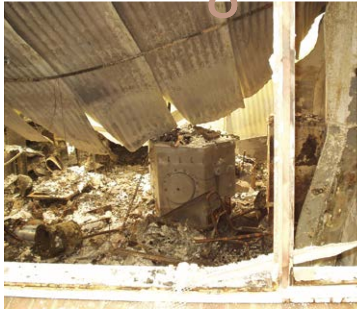
Figure 1. The first incarnation of NIFS, sitting amid the ruins of the detector lab at Mount Stromlo Observatory following the January 2003 bushfire. Photo courtesy of Peter McGregor.
