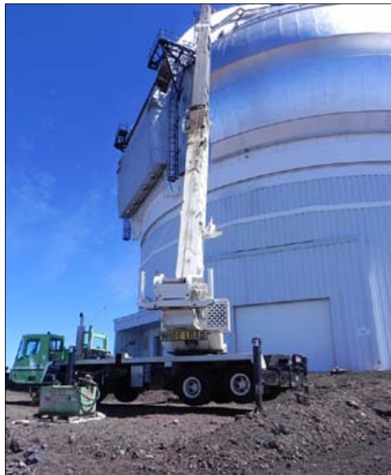
Figure 3. A 150-foot telescoping crane was needed to install the Shutter Service Platform.
