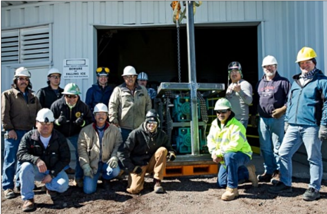
Figure 1. The dome repair team, just before lifting the repaired gearbox back into position.
