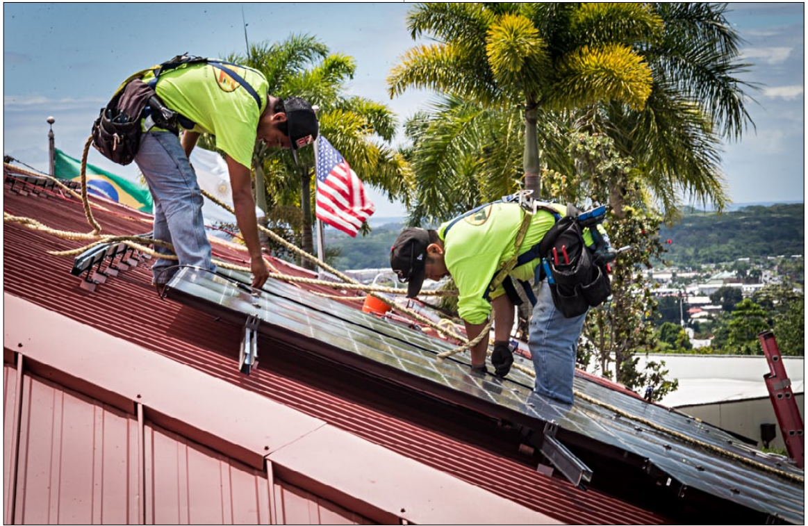
Figures 3-4 Installation of photovoltaic panels on rooftop of Gemini's Hilo Base Facility in Hawai'i (top and bottom).
