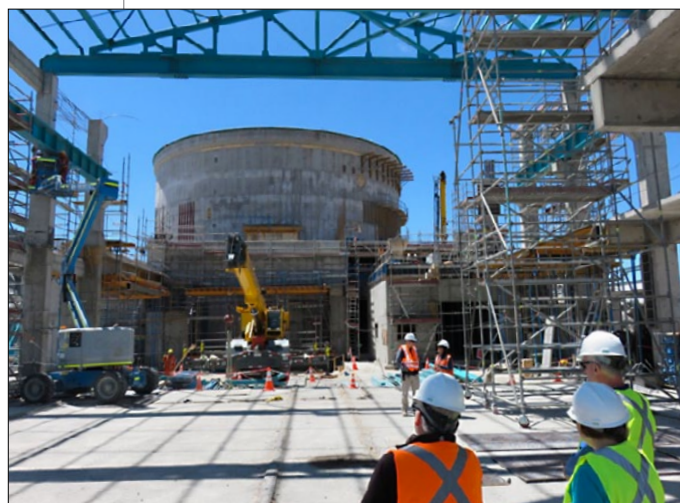
Figure 3. View of the LSST telescope enclosure from where the LSST coating plant will be located.
