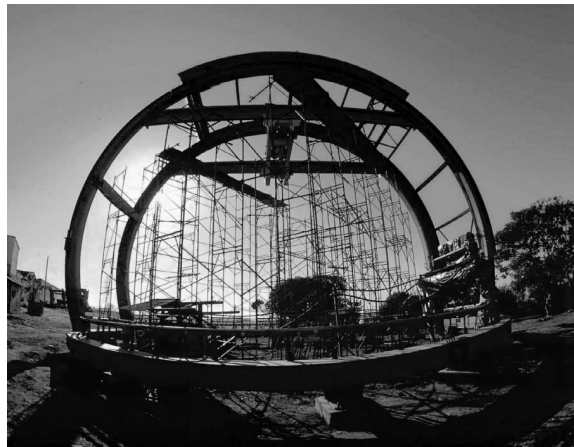
The structural steel work for the dome is seen during the trial assembly at the facility of Equatorial Sistemas, São José dos Campos, Brazil.
