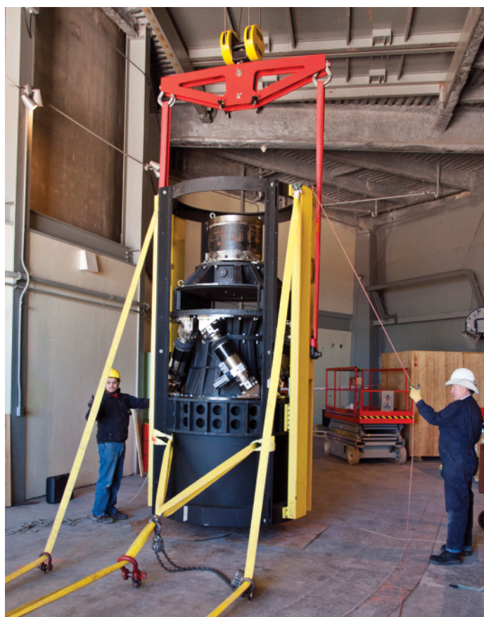
Figure 3: CTIO's DECam installation engineer, Freddy Muñoz (left), and telescope operations manager, Gale Brehmer, assist during a rotation test of the DECam cage loaded with dummy weights to emulate the mechanical behavior of the assembly during installation. (Image credit: Tim Abbott/NOAO/AURA/NSF.)
