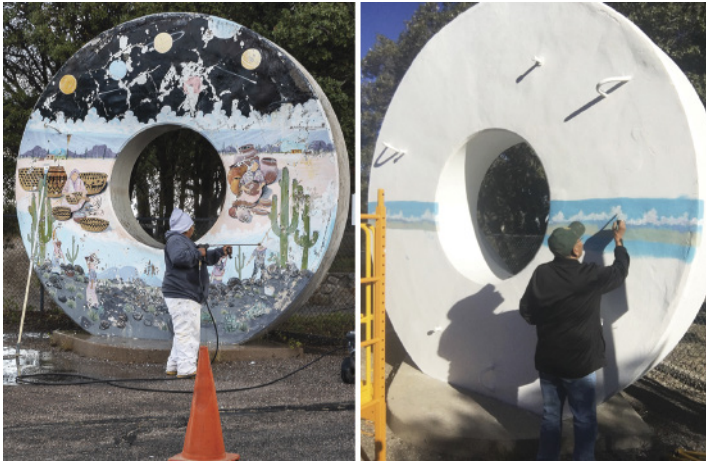
The restoration of the Kitt Peak Visitor Center concrete donut mural. Left to right: Power washing and removing the existing mural (D. Salman/NOAO/AURA/NSF); Artist Michael Chiago begins painting his third mural on the concrete donut (V. Segundo/NOAO/AURA/NSF); Mid-point of mural painting (W. Buckingham/NOAO/AURA/NSF).
